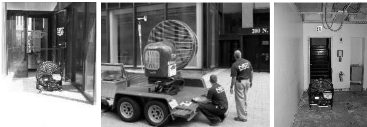
Figure 3. Fan Placements: Portable fan outside, trailer mounted fan and portable fan inside.
